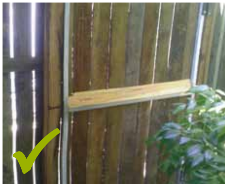
A minimum 60 degree angled wedge along the horizontal rail eliminates a foothold.
