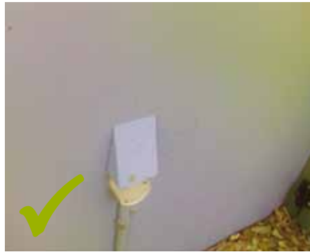
A power outlet has been shielded appropriately.
